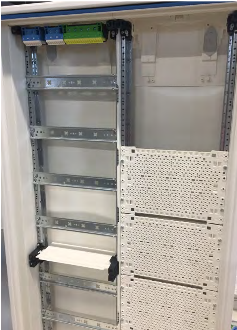
Cabinet with installed partitions
