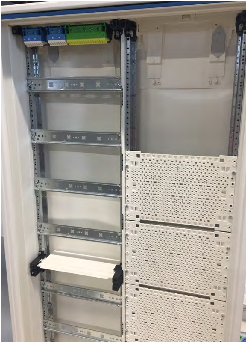
Cabinet with installed partitions
